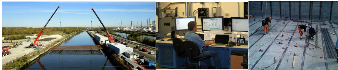
Figure 6: Barrier Construction, Electrodes, and Control Room--Photos by Smith & Root
